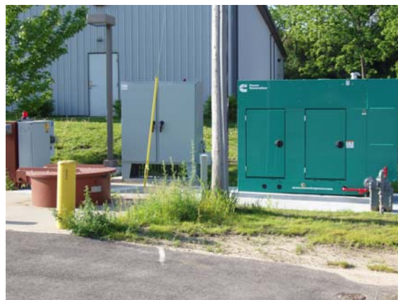
Viaduct Street Lift Station
