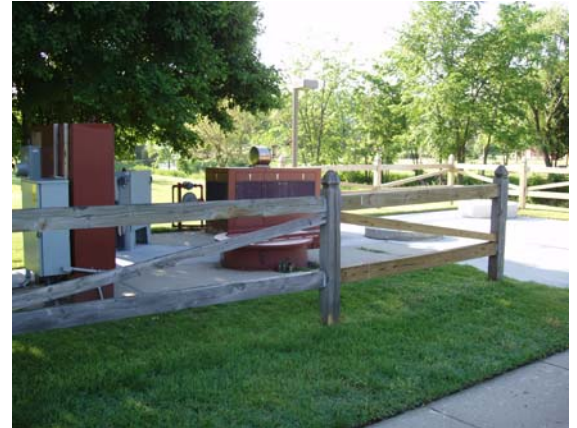
Canal Avenue Lift Station
