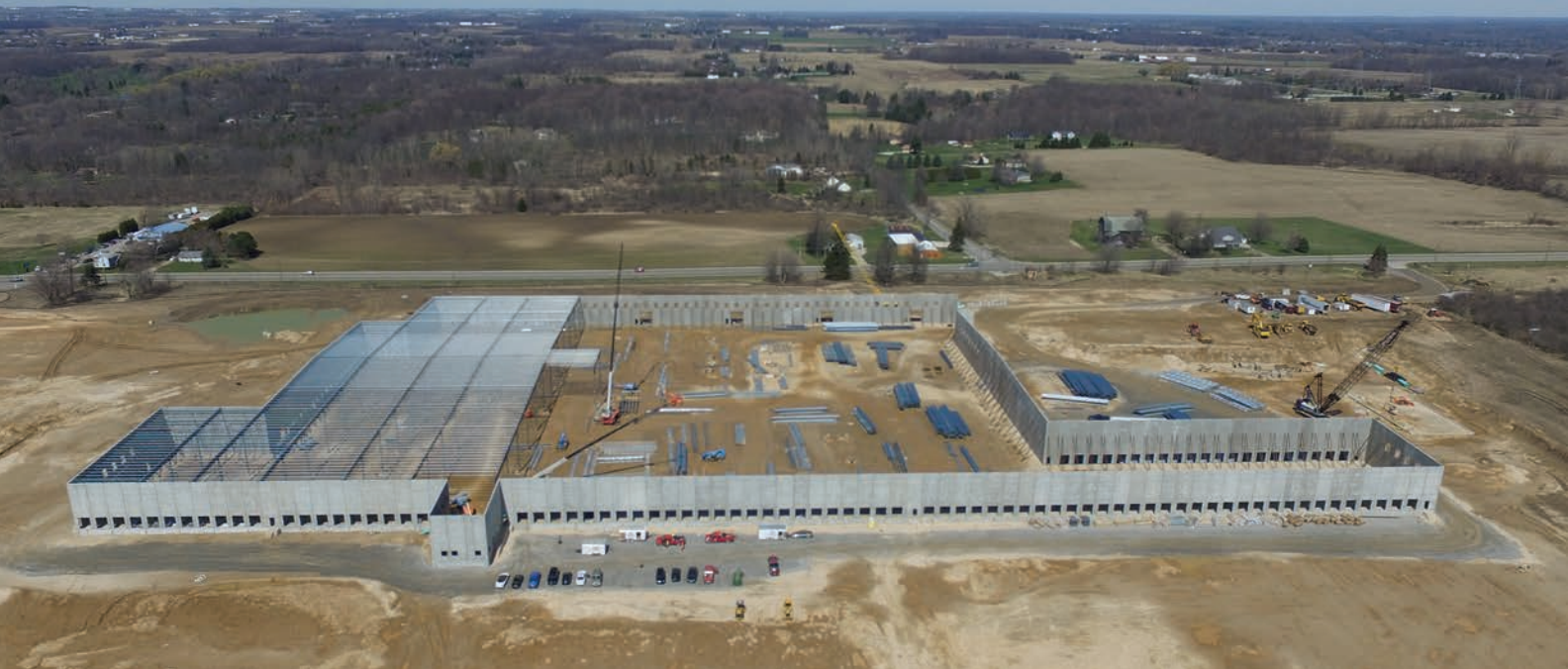
MOORE & BRUGGINK IS PROVIDING CIVIL ENGINEERING SERVICES FOR A NEW 346,000-SQUARE-FOOT FEDEX DISTRIBUTION CENTER LOCATED ON A 60-ACRE PARCEL IN WALKER, MICHIGAN. THE PROJECT BEGAN IN NOVEMBER 2015 AND IS ANTICIPATED TO BE COMPLETED IN FEBRUARY 2017.
