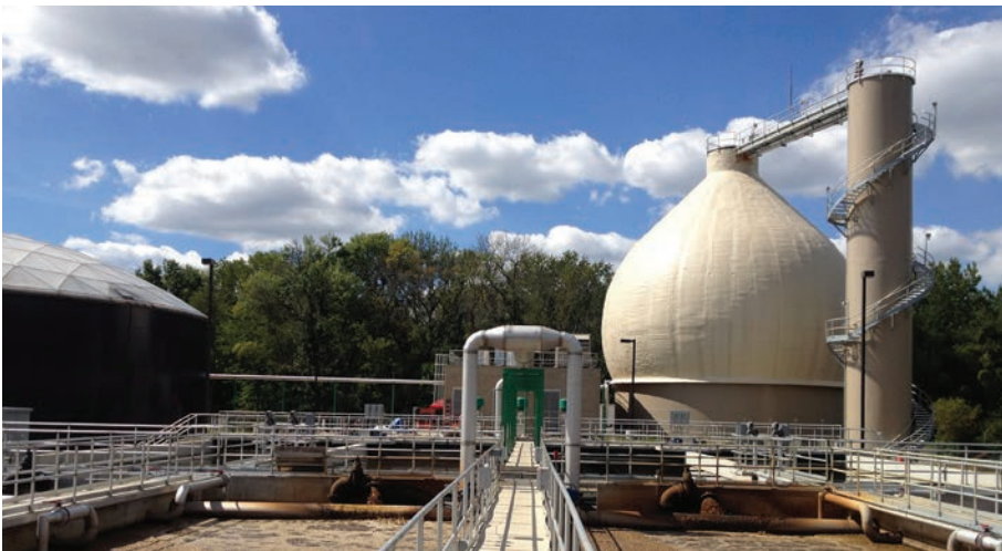
MOORE & BRUGGINK PROVIDED DESIGN AND CONSTRUCTION ENGINEERING SERVICES FOR A MAJOR CLEAN WATER TREATMENT PLANT UPGRADE FOR THE CITY OF GRANDVILLE. THE PLANT INCORPORATES THE STATE'S FIRST EGG-SHAPED ANAEROBIC DIGESTER AND BIOGAS COGENERATION SYSTEM, WHICH WILL CREATE HEAT AND POWER FOR THE PLANT TO OFFSET ENERGY REQUIREMENTS AND SAVE MONEY.
