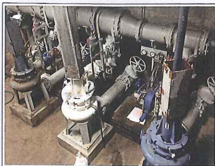
Shafting, coupling guards, seal system, compressor, bearings and hydraulically operated valves required constant maintenance and repair.
