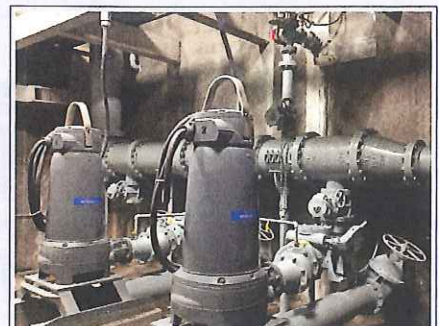
Standard air cushioned check valves and ITT Pumpsmart VFD's allowed for the elimination of the old style hydraulic oil operated valves decreasing complexity of the system.
